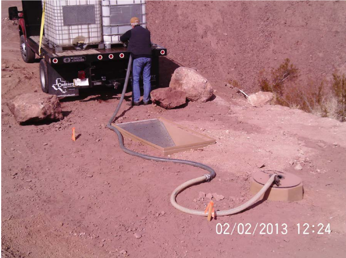
Christian filling up the tank for the sheep that were there watching us during the install
